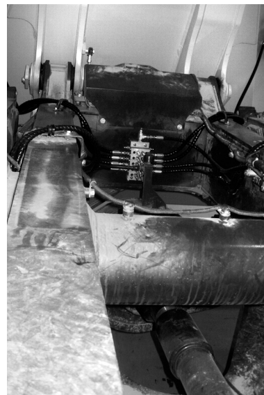
FIG. 115: Rear Secondary MSP Divider Valve
