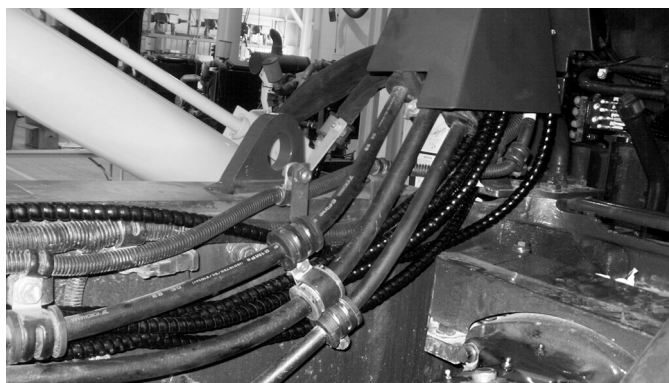
FIG. 107: Hoses left side to left side dump body frame rail on HM300-5.
